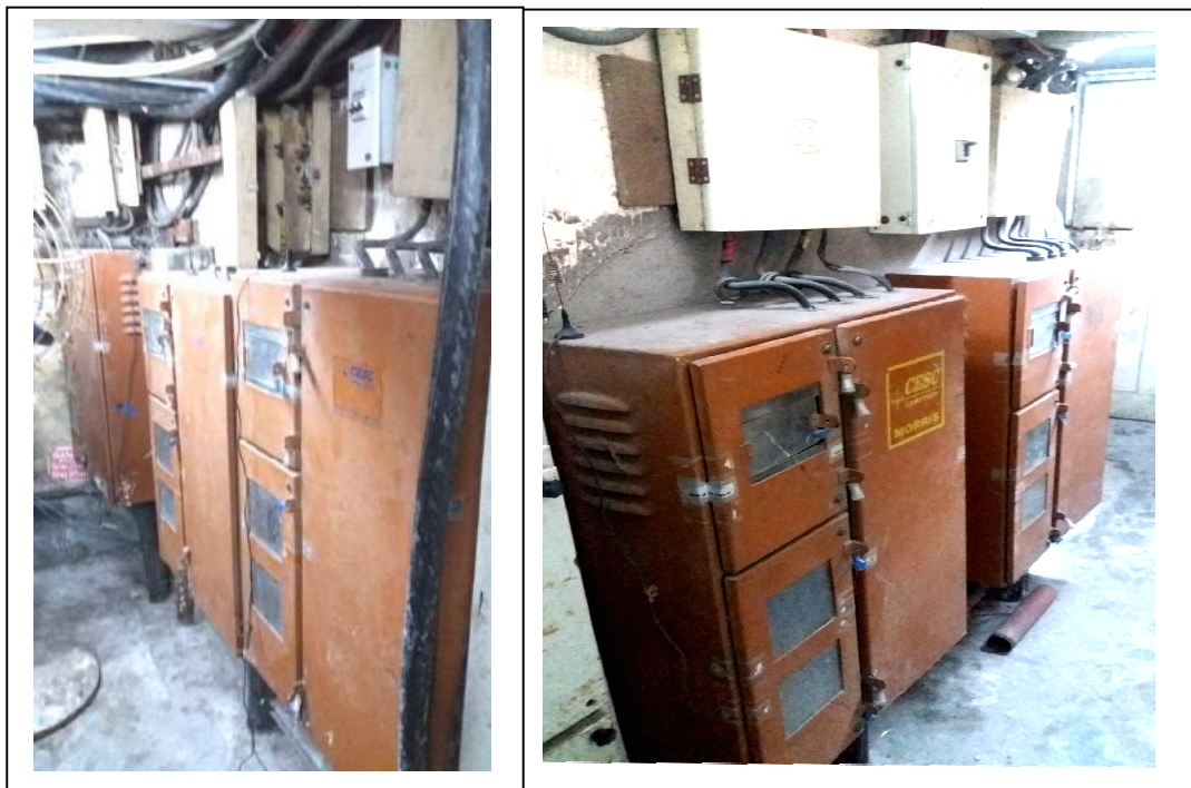
Fig 3.2 Meter in the Panel Room
